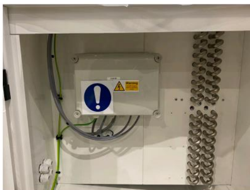
Terminal box for external control cabinet
