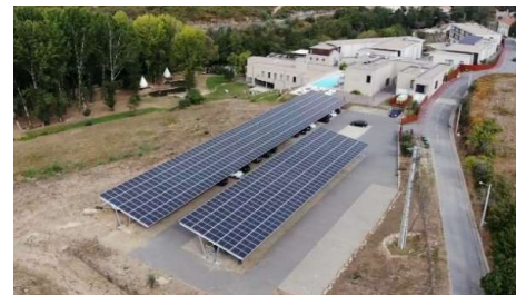
AQUA VILLAGE SPA RESORT Oliveira do Hospital UPAC Carport de 235 kWp
